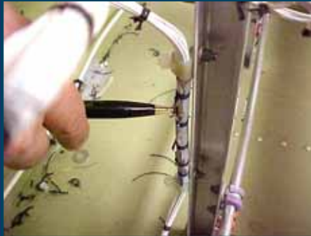
Improperly installed sleeving
