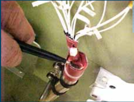
Damaged conduit covering
