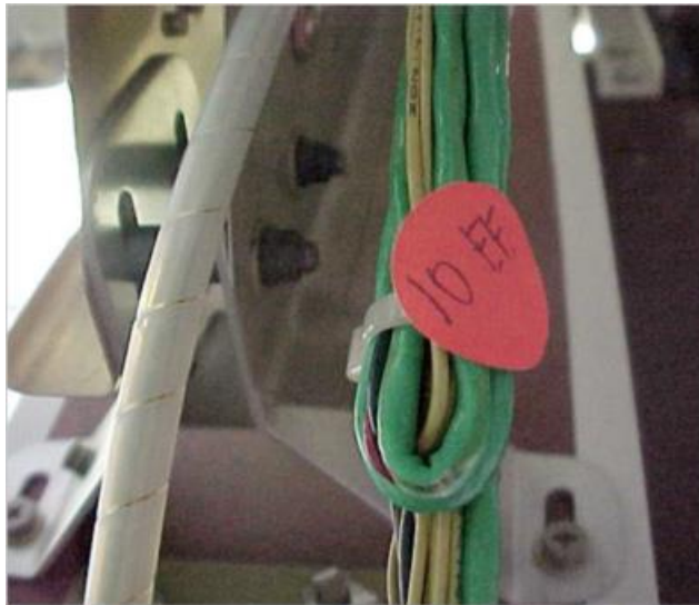
Example of improper bend radius
